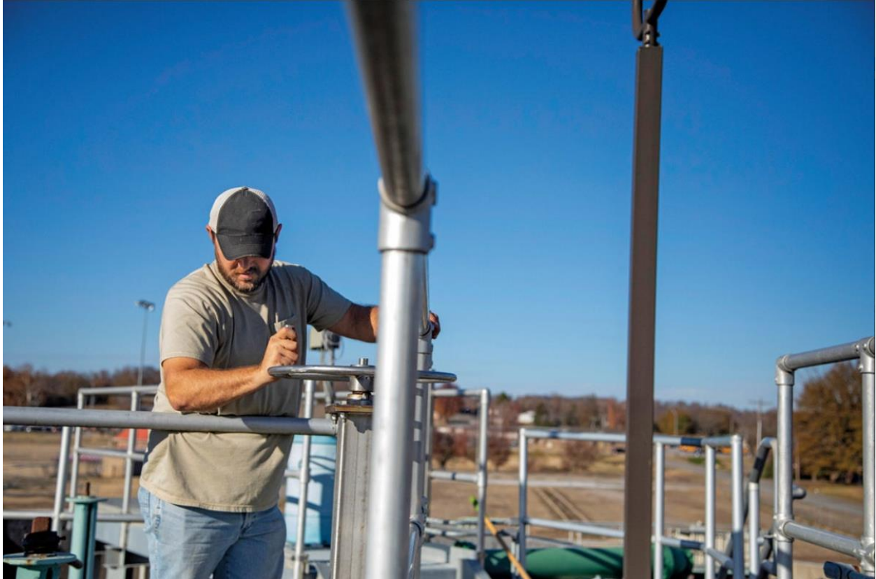
Town of Muldrow (Oklahoma) wastewater operator Josh Randolph adjusts the Digester Skimmer at the wastewater treatment facility in Muldrow. (Photography by David McNeese)
